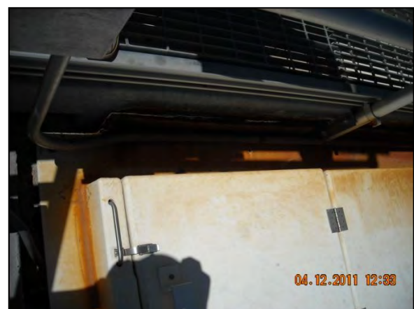
Aerobic Digesters – Covers (2)
