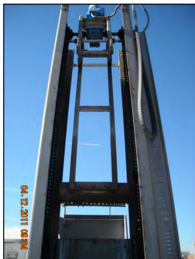
West Mechanical Bar Screen
