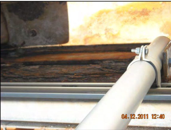
Aerobic Digesters – Covers/Piping Damage (2)
