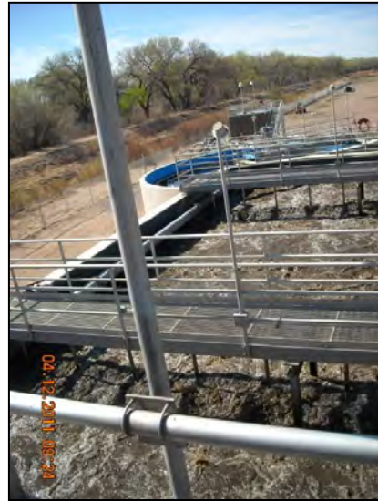
East Aeration Basins
