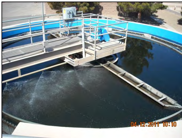
West Secondary Clarifier
