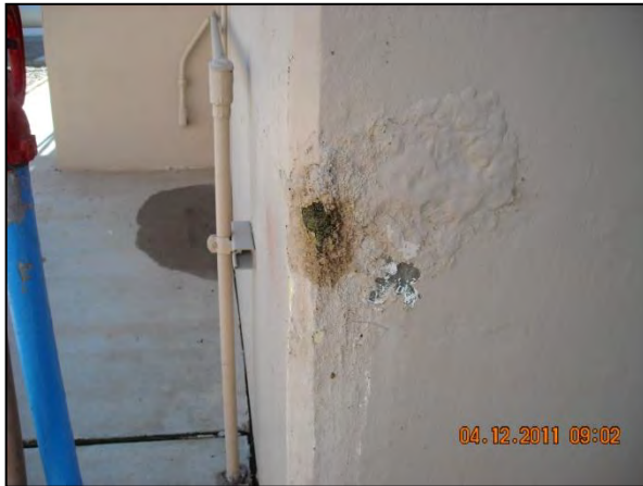
Damage on Grit Chamber Wall
