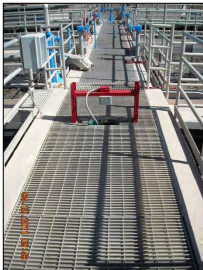
Aeration Basins RAS channel (Under Grating)
