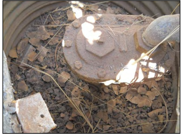
Air Relief Valve in Pressure Manhole
