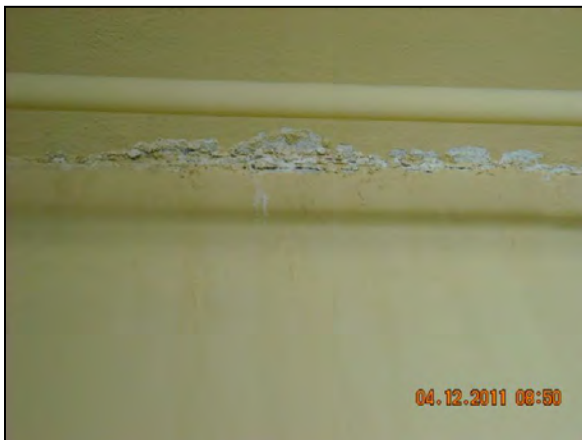
Damage Inside Grit Pumps Room
