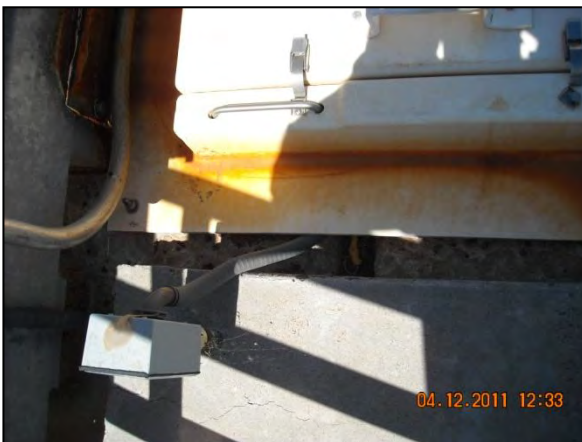
Aerobic Digesters - Covers (1)
