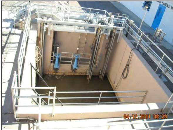
Influent Lift Station
