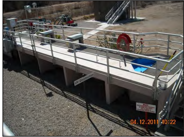
UV Disinfection System
