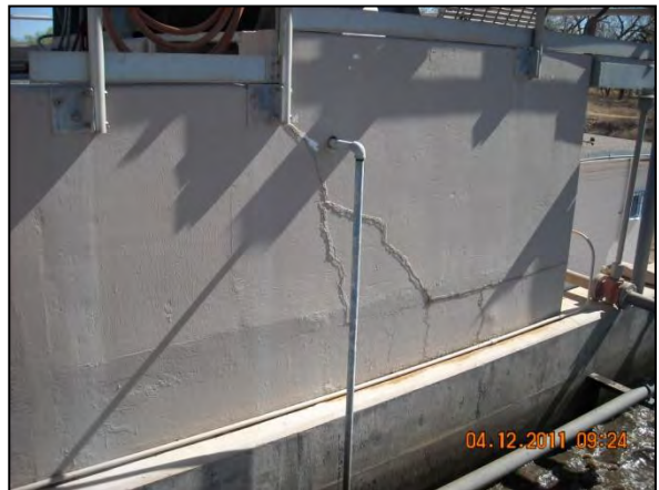
Damage on Wall at Entrance Works Structure
