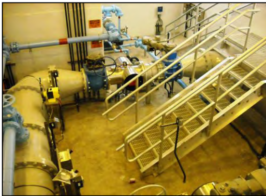
In-Vessel UV Disinfection
