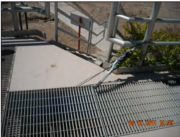
External Support for the Weighted Effluent Weir
