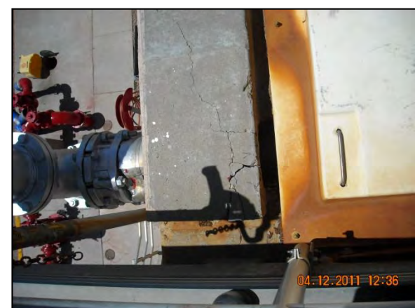
Aerobic Digesters – Covers/Concrete Damage (1)
