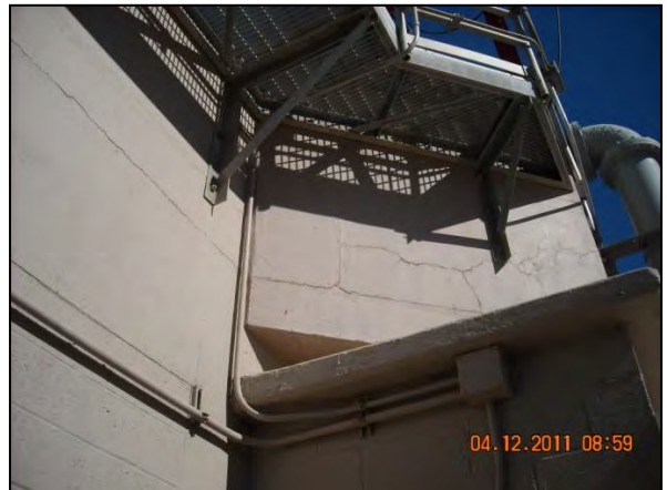
Damage Outside Grit Pumps Room
