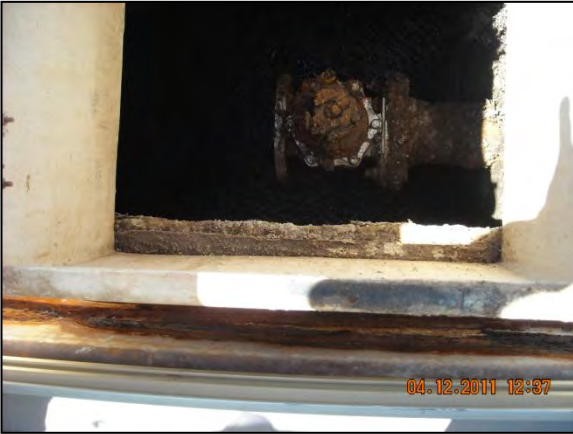
Aerobic Digesters – Piping Under Covers
