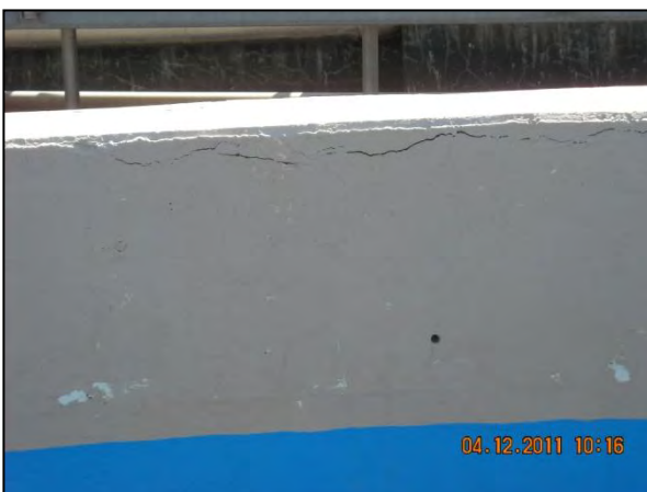
East Secondary Clarifier Damage on Concrete
