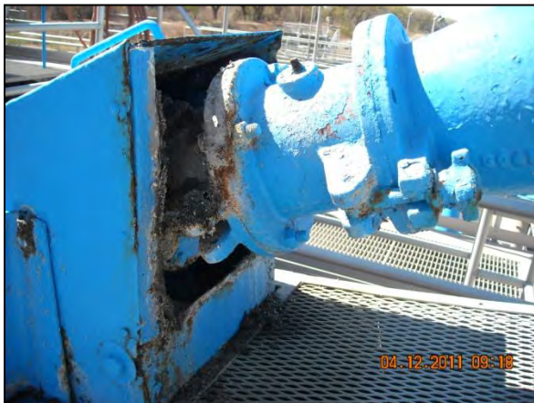
Damage on Cyclone/Grit Classifier
