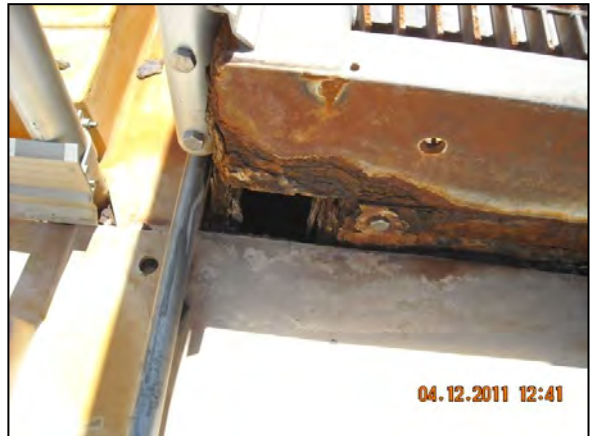
Aerobic Digesters – Covers/Piping Damage (2)
