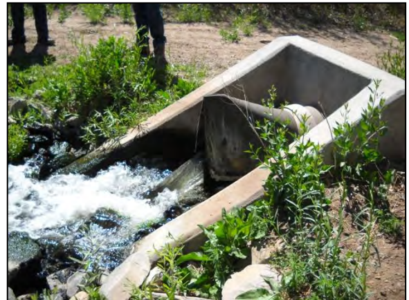
Discharge of Treated Effluent
