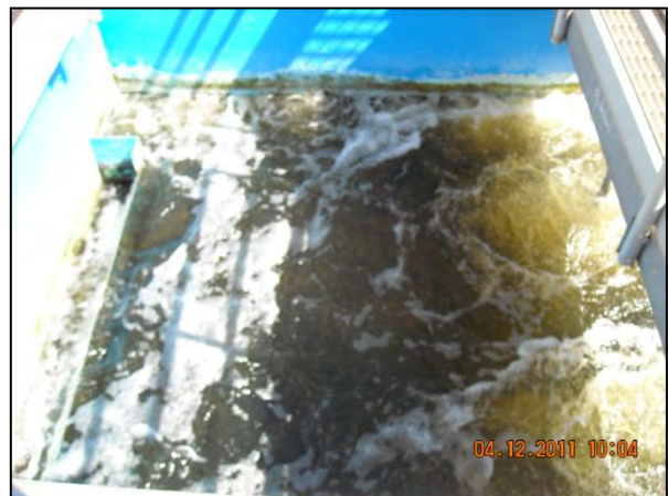
Clarifier Effluent Re-aeration Box
