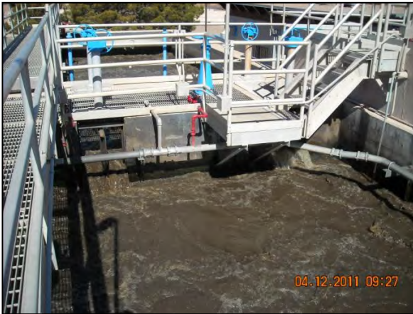
Aeration Basins Influent Gates (Significant Corrosion)
