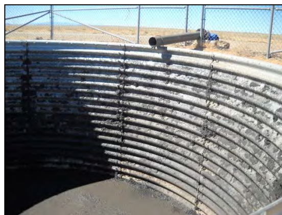
Sludge Nursing Tank
