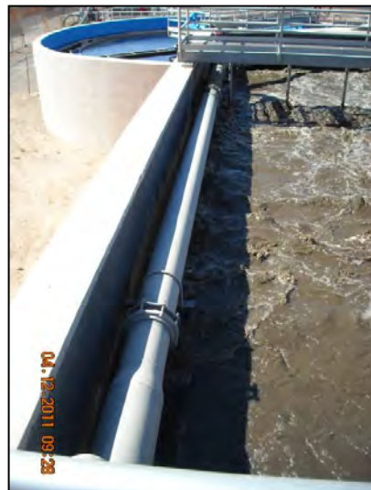
East Aeration Basins Air Piping (Pipe May be Leaking)
