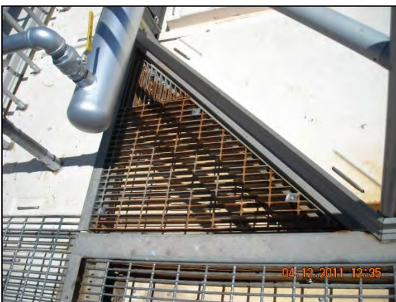
Aerobic Digesters – Walkways/Grating
