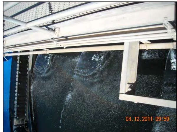
East Secondary Clarifier Spray Bar
