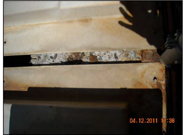
Aerobic Digesters – Covers/Concrete Damage (2)
