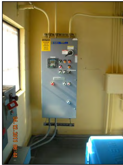
VFDs for Influent Pump
