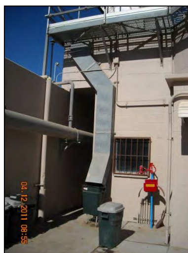
Bar Screens Discharge Chute
