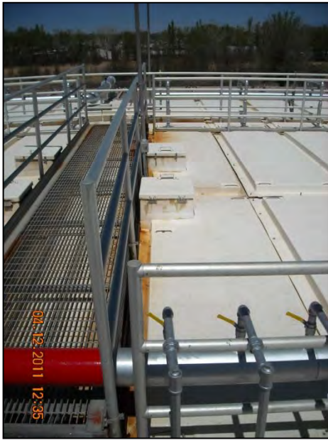
Aerobic Digesters - Covers and Walkway
