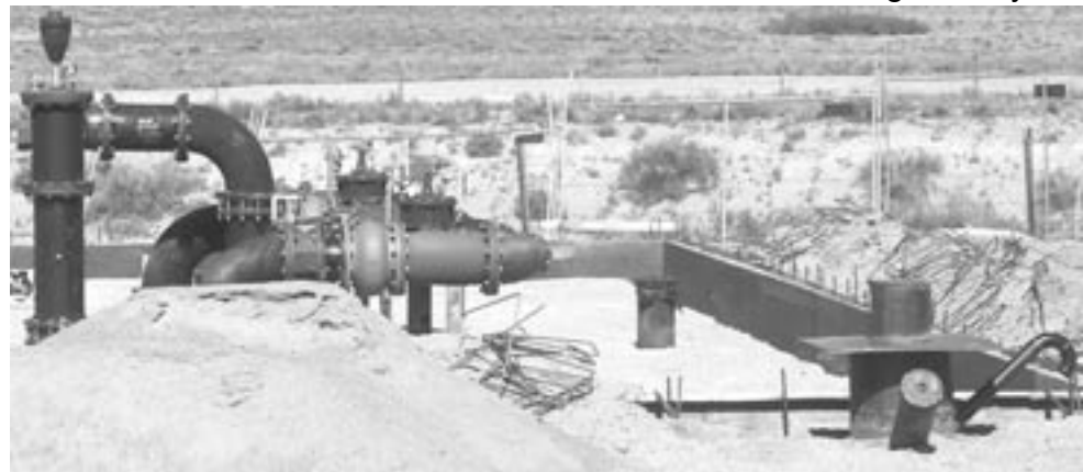
Well #6 pump house piping takes shape in the desert. When the piping is complete, the foundation will be poured. At the far right is the well site. This is part of the water loop project that provides more efficient service and better fire protection in the village.
